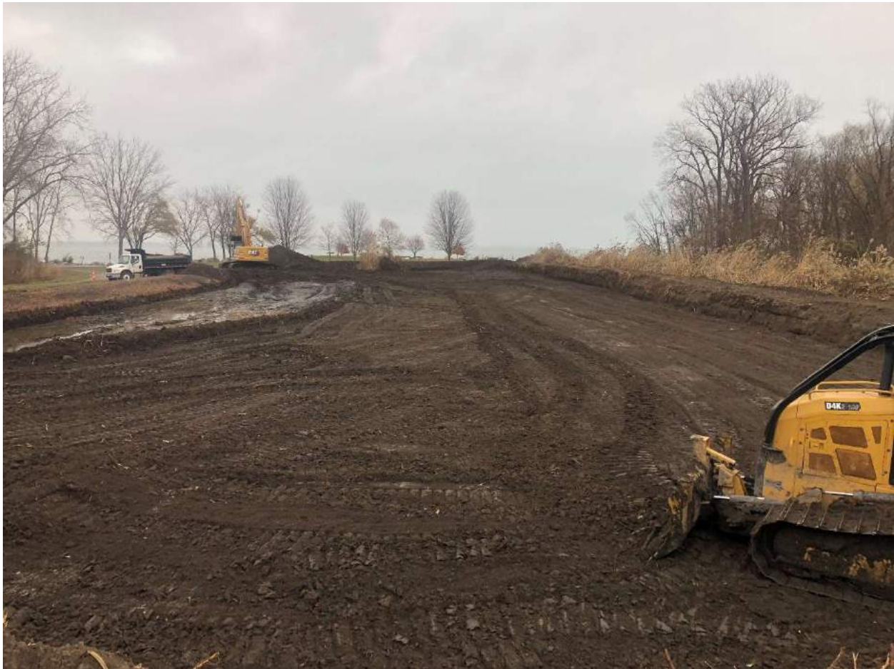
Figure 2: At Lake Erie Metropark, a pile of dredged materials has been excavated and transported to a designated storage location within the park. This excavation cleared this site, adjacent to the marina, and will allow dredge activities to move forward in early 2024.
