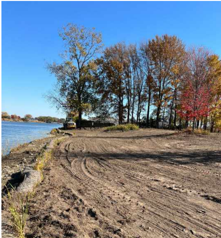
Figure 1: At Lake St. Clair Metropark, Natural Resources staff completes finish grading and preparation for seeding at the shoreline restoration project site. This site will be seeding in December 2022.
