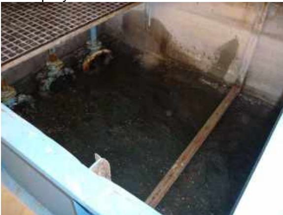
Wave pool surge pit
