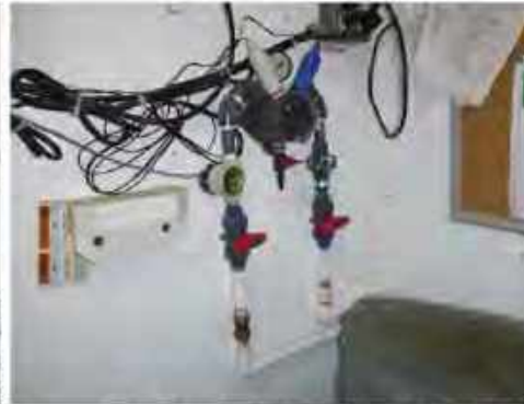
Image 76: Chemical Controller Wiring & Sample Cell
