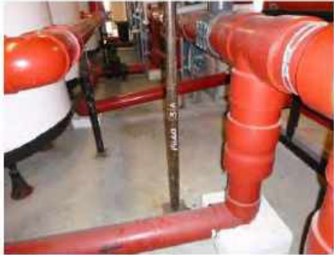
Image 39: Mechanical Room Piping with Concrete Thrust Blocks
