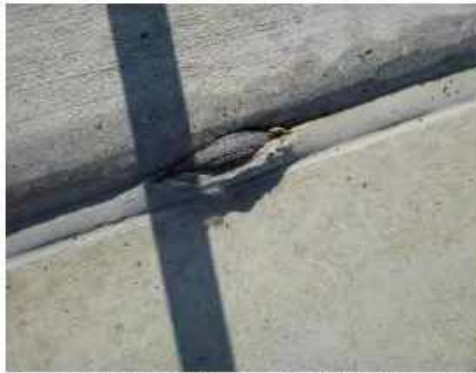
Image 34: Deteriorating Deck Sealant and Exposed Joint Backing
