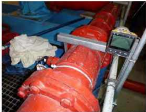
Image 43: Digital Flow Meter Display & Sensor
