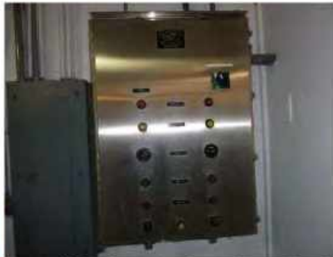
Image 60: Recirculation Pump Starter Panel
