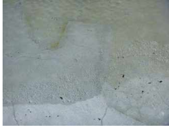
Minor cracking and pitting of the pool surface
