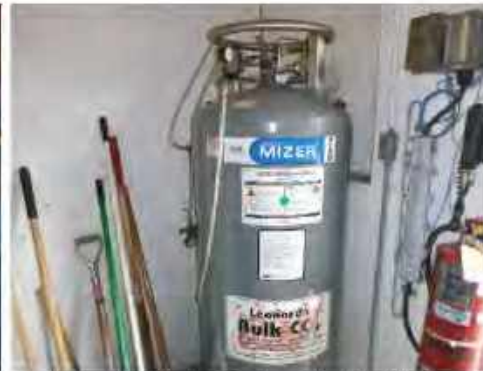
Image 68: Bulk Carbon Dioxide Tank
