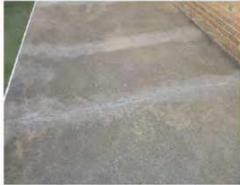
Image 33: Deck Cracking at Wave Caissons
