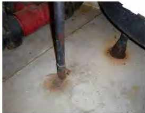
Image 50: Corrosion at Filter Support Leg
