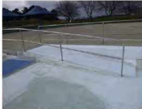
Image 21: Noncompliant ADA Ramp Entry
