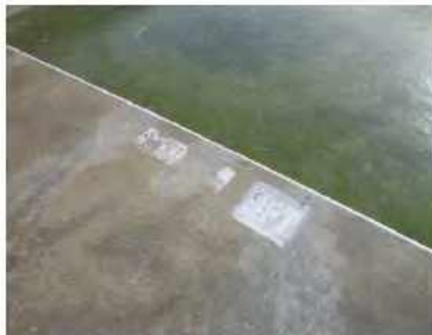
Image 28: Faded Painted Deck Markings
