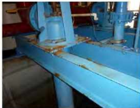
Image 64: Corrosion at Coated Steel Surge Tank
