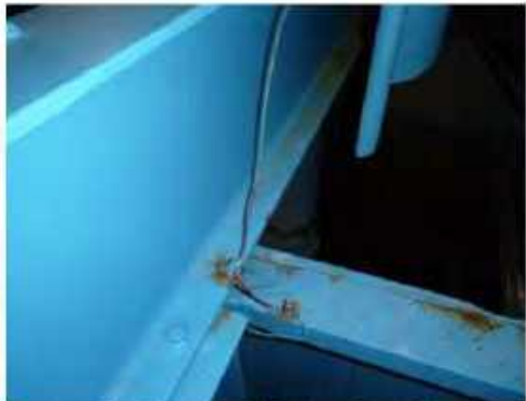
Image 59: Wave Pool System Bond Wiring
