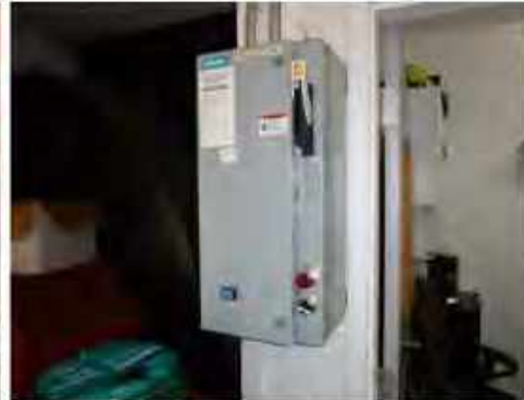
Image 62: Sprayground Pump Starter
