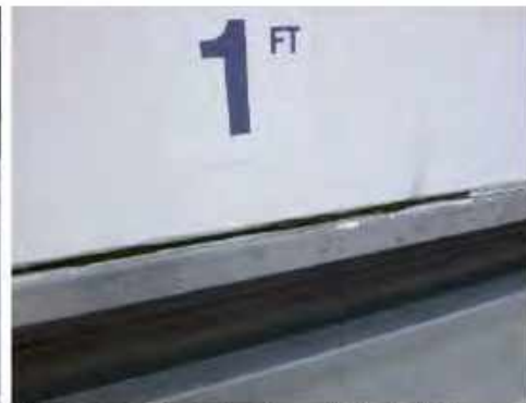
Image 16: Deterioration of Sealant Above Gutter and Concrete
