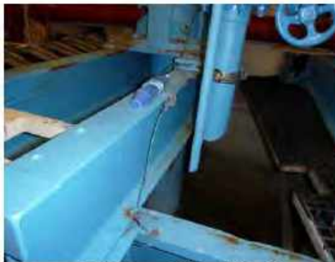
Image 65: Make-up Water Fill at Surge Tank
