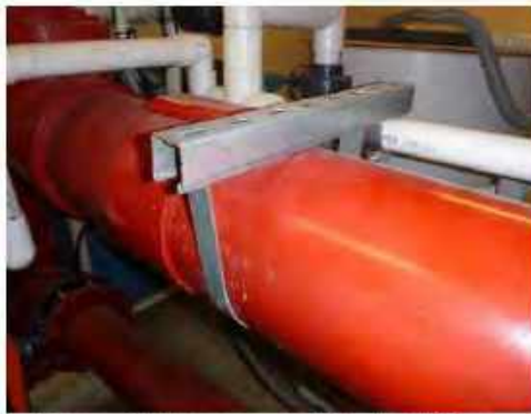
Image 47: Unsupported Strut and Pipe Guides / Straps
