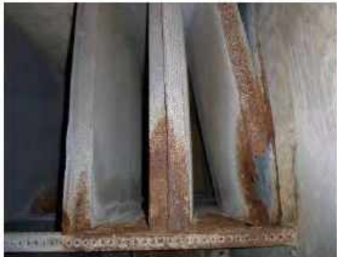
Image 82: Corroded Baffles in Equipment Room
