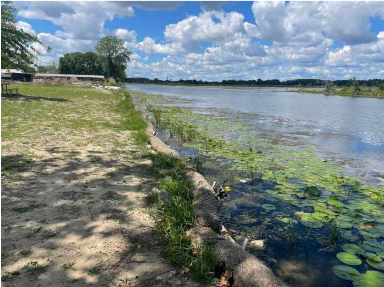
Figure 1: At Lake St. Clair Metropark, the current condition of the shoreline on the Black Creek Marsh. This shoreline will receive final grading, seeding, and covering with erosion blanket in the fall of 2022.
