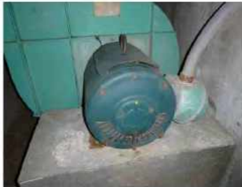
Image 83: Motor and Unsupported Fan
