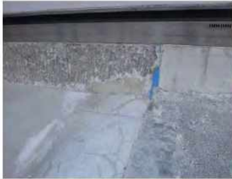
Image 5: Finish & Substrate Deterioration at Expansion Joint
