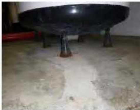
Image 51: Corrosion at Filter Support Legs and Discoloration Likely from a Leak
