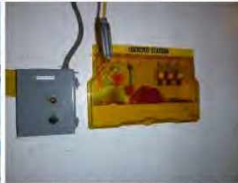
Image 87: Water Level Control Panel
