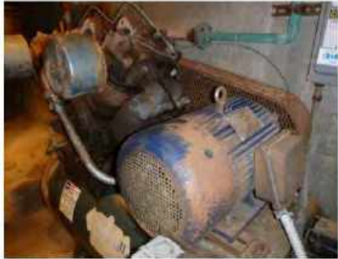
Image 80: Corroded Wave System Air Compressor
