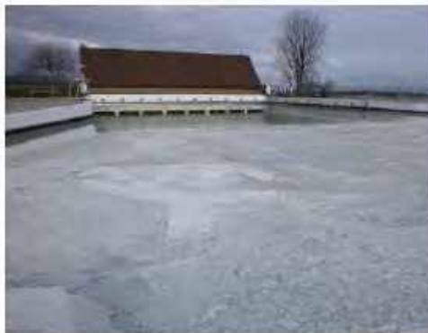
Image 1: Wave Pool Deteriorated Finish & Substrate
