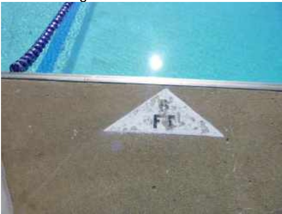
Damaged depth marker
