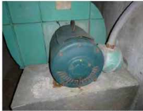
Image 83: Motor and Unsupported Fan
