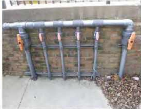
Image 46: Sprayground Feature Manifold
