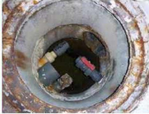
Image 40: Waste Pit Valves
