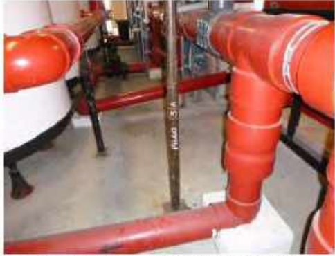
Image 39: Mechanical Room Piping with Concrete Thrust Blocks
