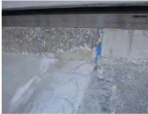
Image 5: Finish & Substrate Deterioration at Expansion Joint
