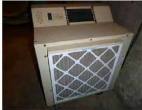
Image 81: Dehumidifier for Wave Pool Equipment Space
