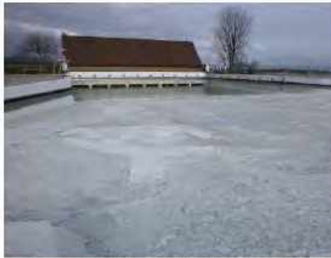
Image 1: Wave Pool Deteriorated Finish & Substrate
