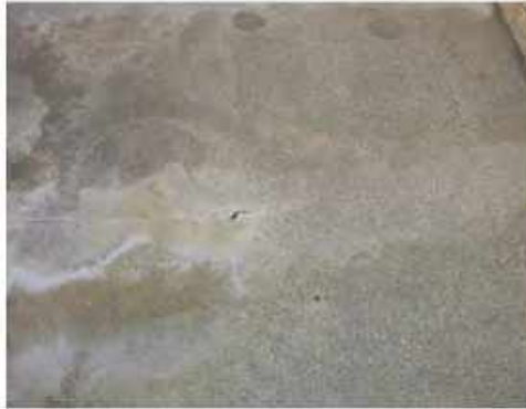
Image 32: Deck Discoloration Likely from Standing Water
