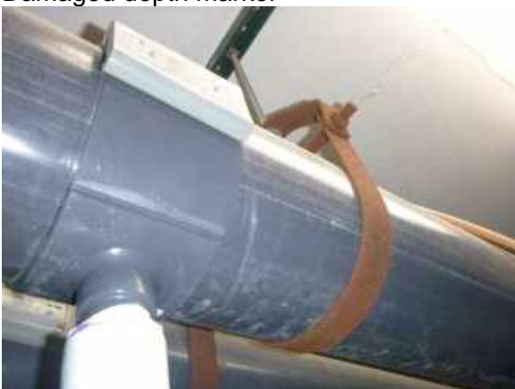
Corroded pipe hanger
