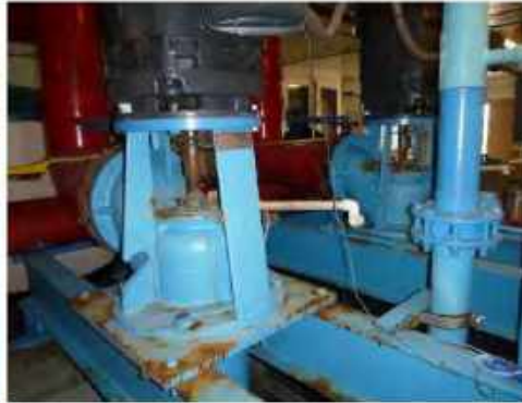
Image 56: Corrosion at Recirculation Pump Base and Frame
