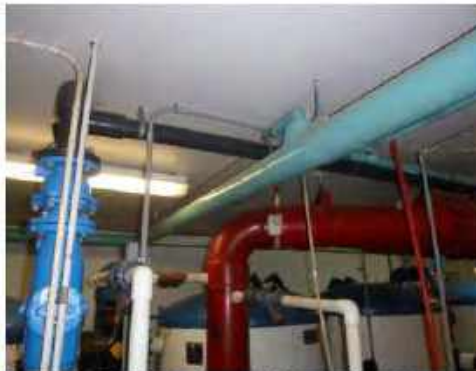
Image 73: Chlorinator Side Stream Taps
