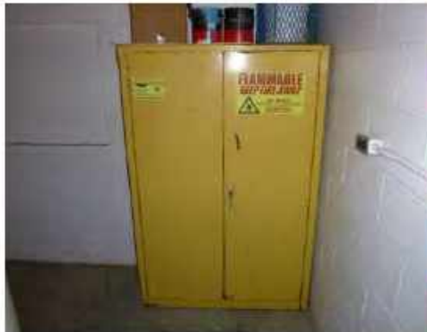
Image 71: Chemical Storage Closet
