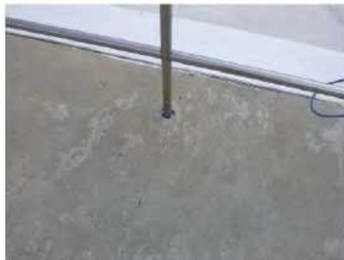
Image 36: Hairline Cracking at Railing Anchor
