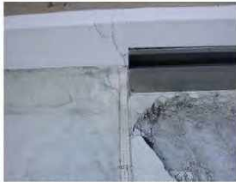
Image 2: Crack Propagating from Termination of Expansion Joint at Gutter
