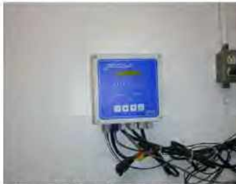
Image 75: Water Chemistry Controller
