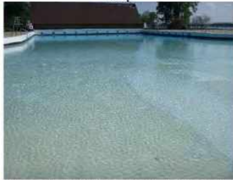
Image 8: Finish Condition in Submerged and Operating Condition
