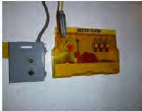
Image 87: Water Level Control Panel
