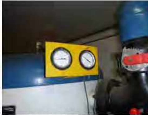
Image 53: Filter Gauge Panel
