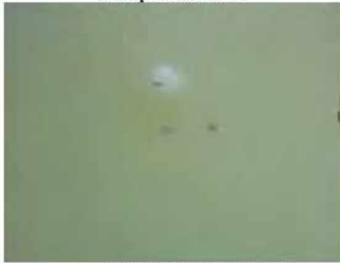
Image 7: Finish Discoloration & Degradation
