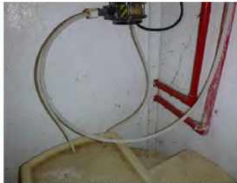
Image 74: Acid Feed Pump and Poly Piping
