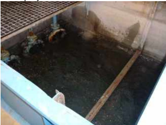
Wave pool surge pit
