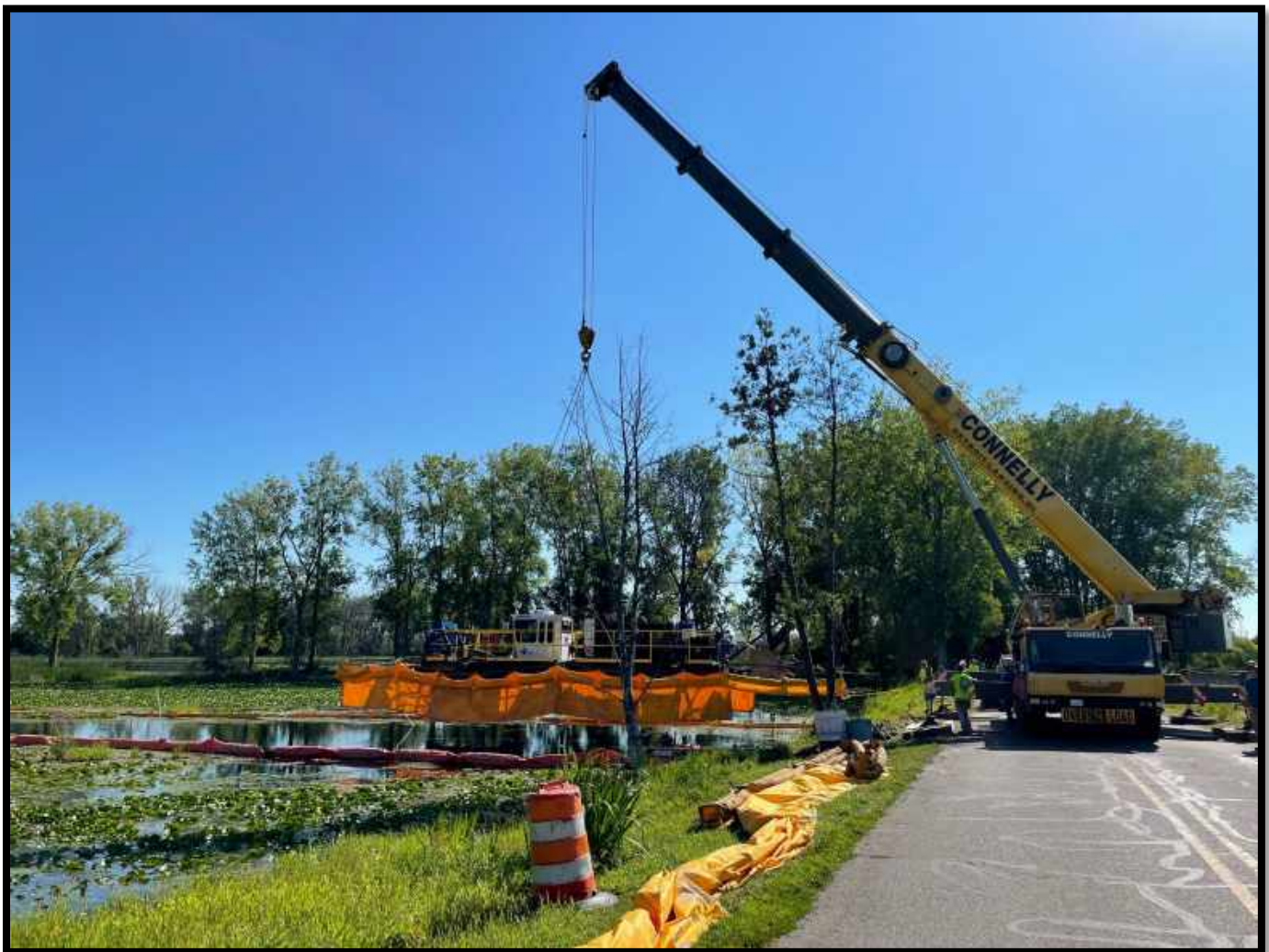
Figure 1: At Lake Erie Metropark, a crane lifts a dredging barge directly into the marsh. This marsh is being dredged as part of a restoration to maintain waterflow, habitat, and paddling access to the area in low-water conditions.
