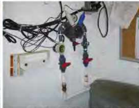
Image 76: Chemical Controller Wiring & Sample Cell
