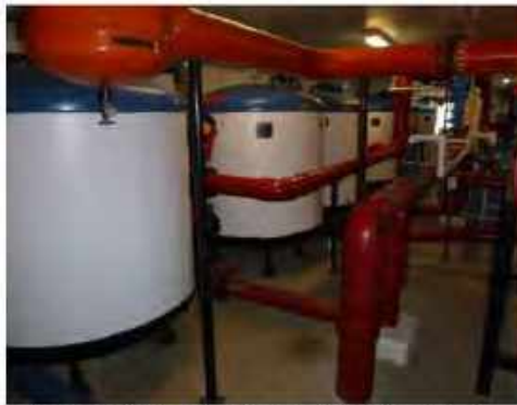
Image 49: Vertical Sand Filtration Tanks
