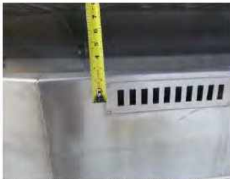
Image 15: Surge Weir and Gutter Hand Hold
