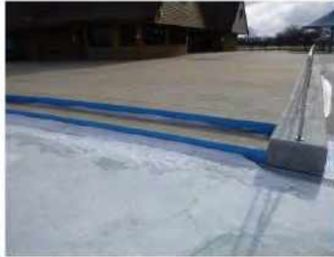
Image 6: Hairline Surface Cracking at Step Entry
