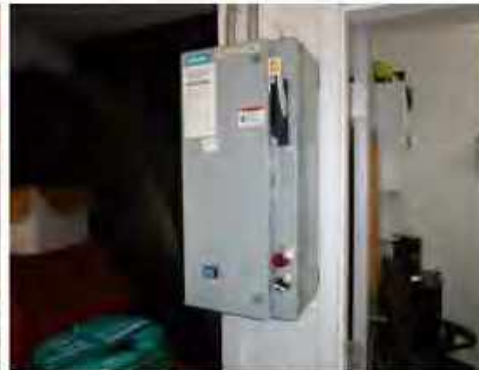
Image 62: Sprayground Pump Starter
