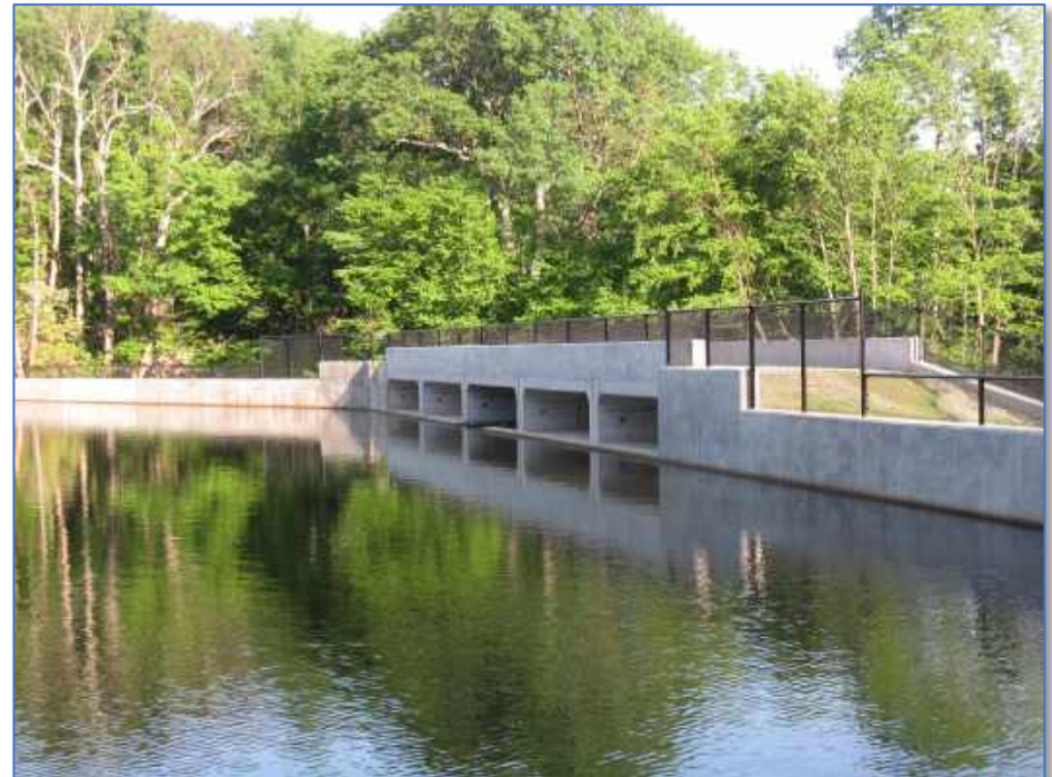
Rehabilitated dam, with box culvert spillway/bridge to resolve significant spillway deficiency and enhance hiking trail access around the lake
