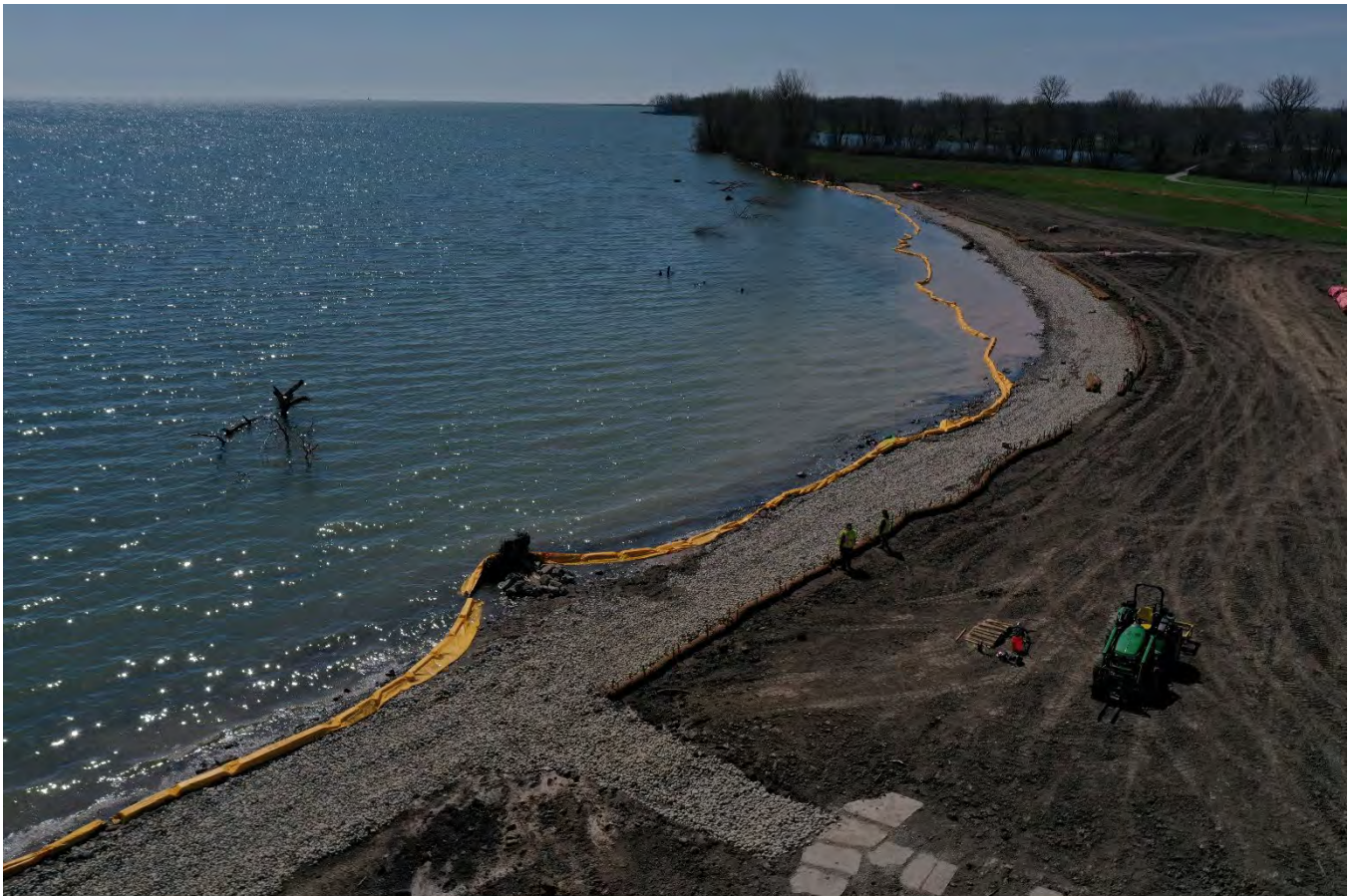
Figure 2: Shoreline restoration project at Lake Erie Metropark has been completed. This aerial drone photo shows the extent of the project area, the newly installed pebble beach, ledgestone access pathways, and regraded area that has been seeded and covered with erosion control blanket.
