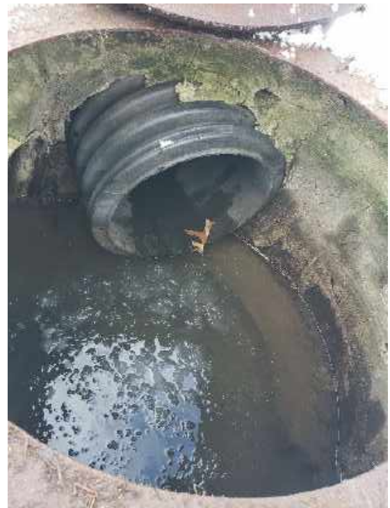
Exhibit 2. Example inlet draining to standing water. If standing water can be avoided, sample from the inlet.
