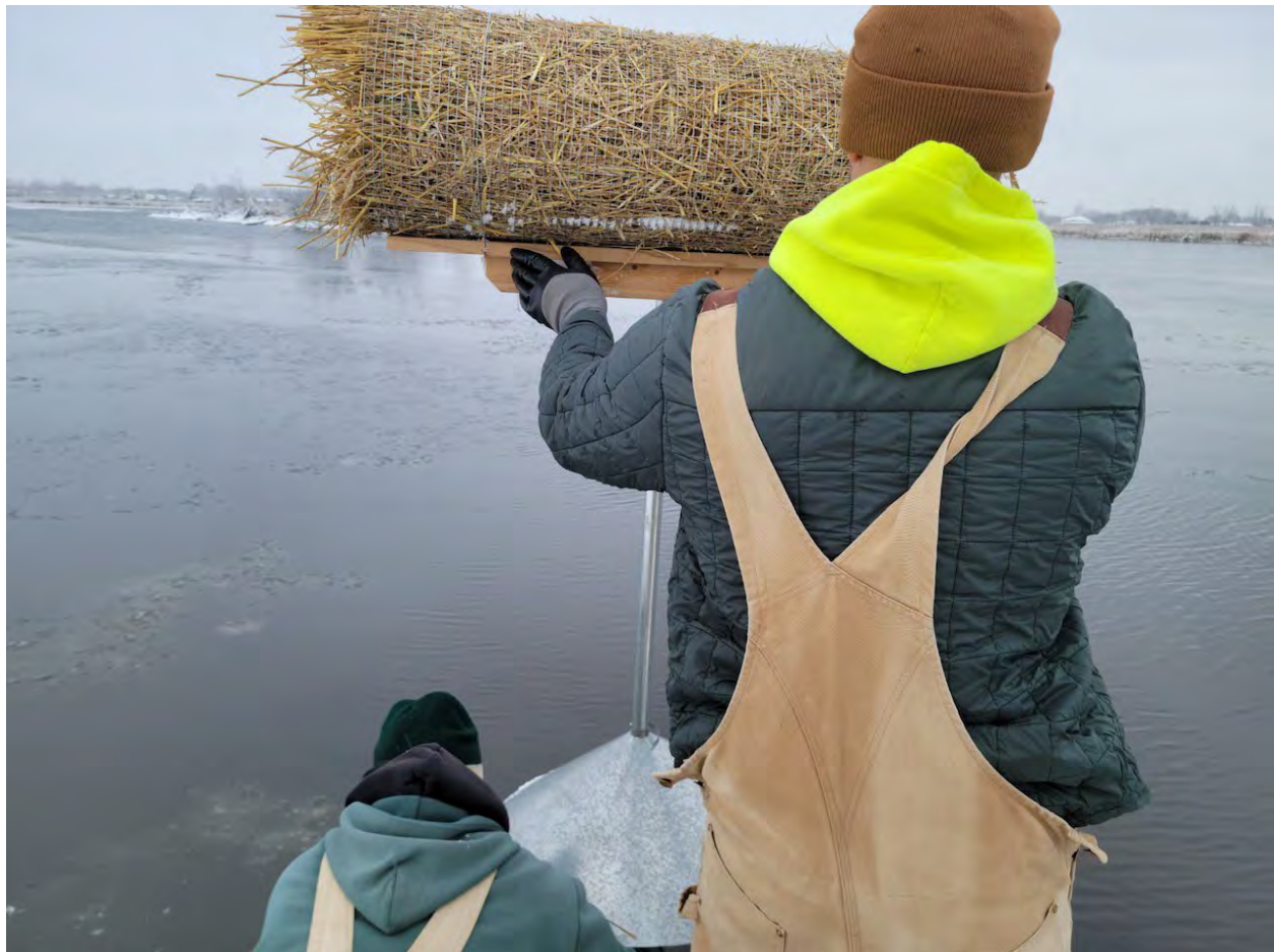
Figure 4: Natural resources staff install mallard and wood duck nesting habitat at Lake St. Clair Metropark. This nesting habitat is part of the Shoreline restoration project funded by U.S. Forestry Service and GLRI.
