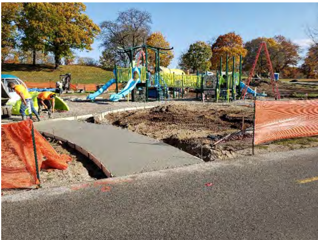
Kensington Accessible Playground (Maple Beach)
